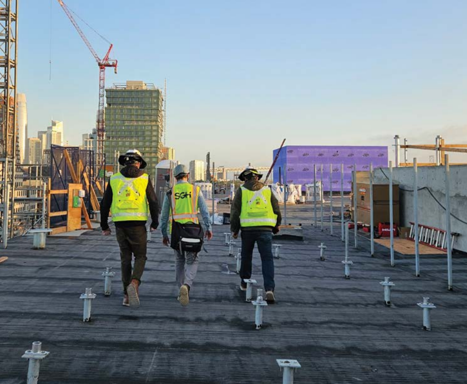
Roof installation site visit at 400 China Basin Street, a multi-family housing project located in San Francisco.
