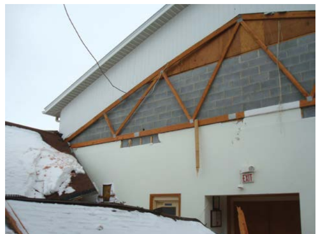
Failed wood truss roof structure due to snow drift accumulation at step in roof height. PHOTO COURTESY WISS, JANNEY, ELSTNER ASSOCIATES
