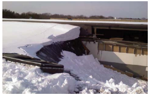
Roof collapse due to snow drift accumulation at the roof height transition. PHOTO COURTESY WISS, JANNEY, ELSTNER ASSOCIATES
