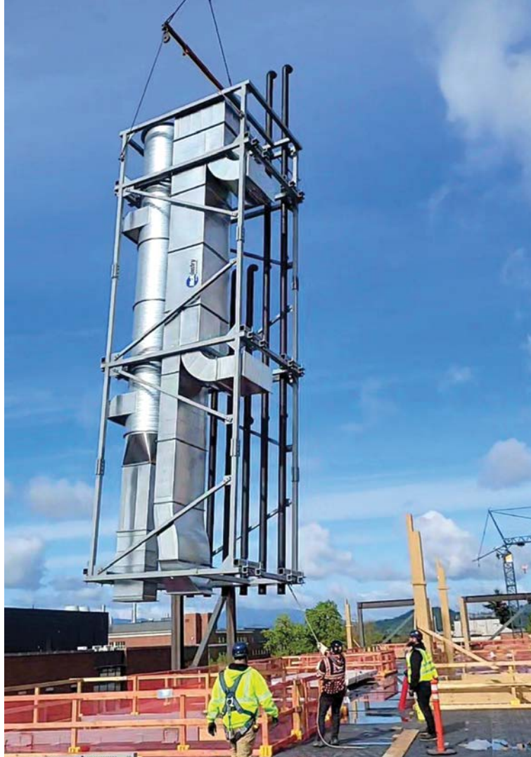
Oregon State University's Jen-Hsun Huang and Lori Mills Huang Collaborative Innovation Complex utilized a vertical, prefabricated multi-trade rack for the mass timber structure's ductwork and piping, which eliminated weeks of potentially hazardous on-site labor. PHOTO COURTESY MCKINSTRY
