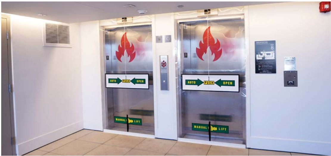
These seals on elevator openings in this data center prevent smoke from spreading in multi-floor facilities, ensuring clear paths for occupants and first responders.
