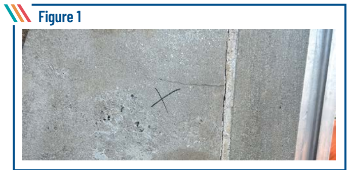
Figure 1 Incipient spalls on the exposed face were identified visually, and the units were marked out for replacement.
