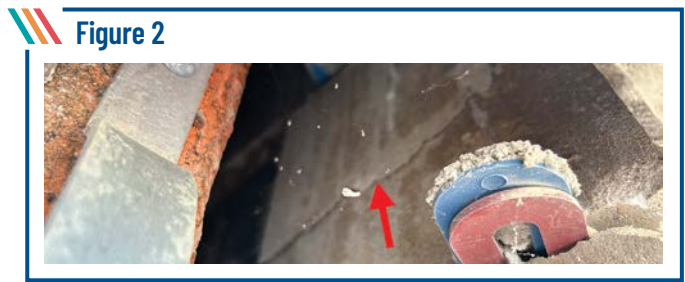
Figure 2 After removal of the units with damage on the exposed face, adjacent units were visible within the wall cavity, and numerous cracks and spalls were discovered on the back face (arrow).
