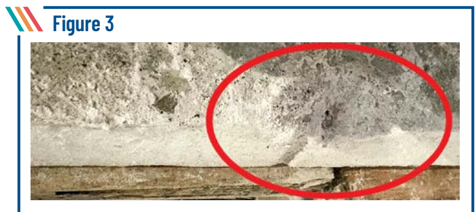
Figure 3 Removal of a few representative marble cladding panels revealed that many panels had spalled on the reverse face at the locations of pin anchors (circle).
