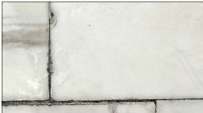
Figure 1: Due to a lack of any expansion joints in the system, the marble floor tiles exhibited chipping and spalling along their edges, where confined by relatively hard mortar joints.
